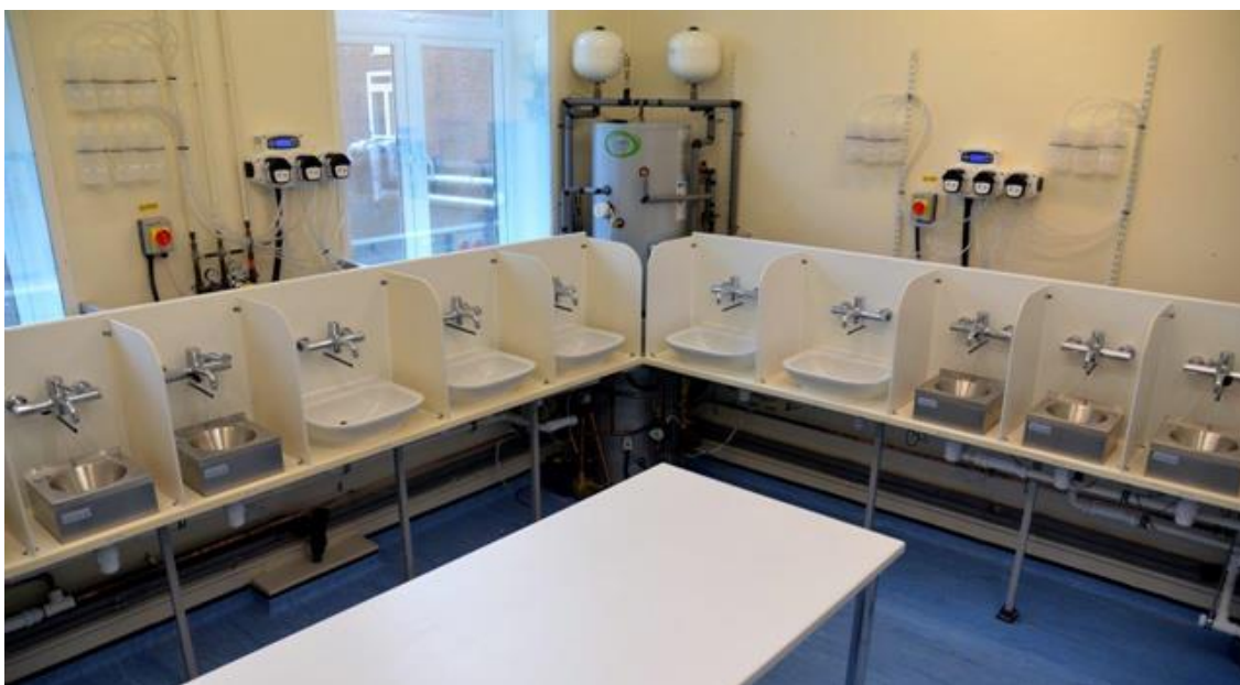
Figure 1: Experimental model system to study the role of the hospital sink in transmission of infection. Taps and drainage are automatically controlled via a building management system.
