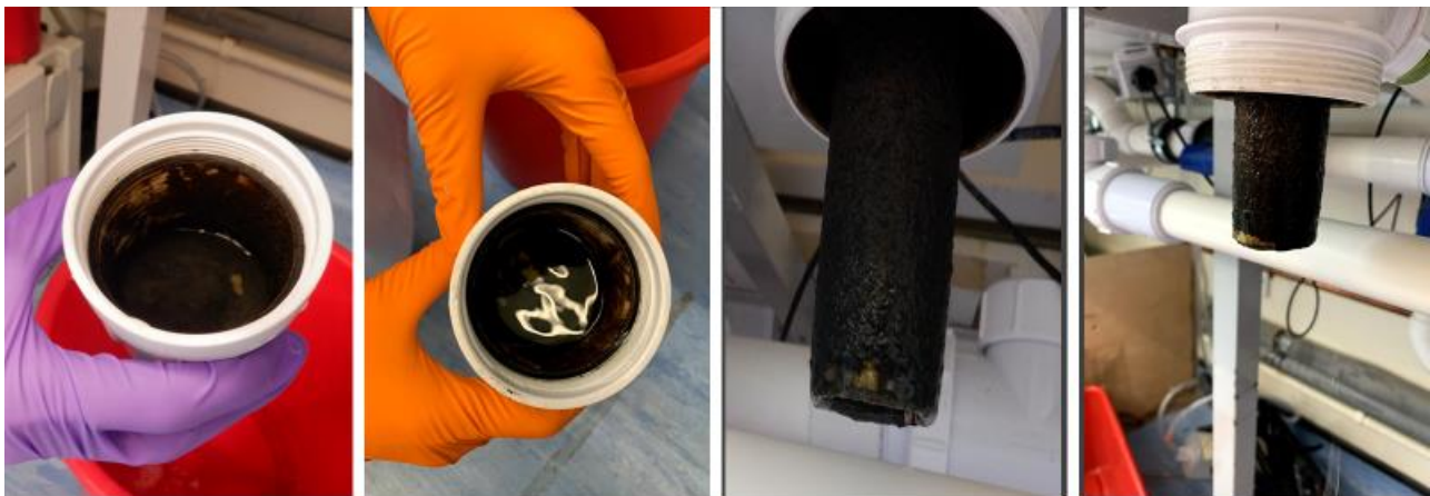
D. Base-draining sink: before and after treatment with a peracetic acid-based foaming disinfectant
