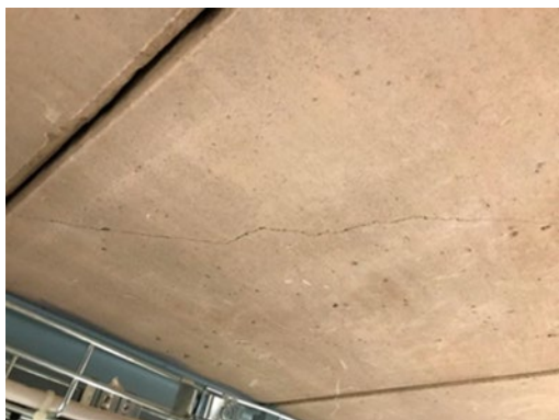
Figure 3.12 - Soffit cracks caused by plant loading above
