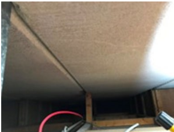
Figure 3.4 - Differential deflection between RAAC planks
