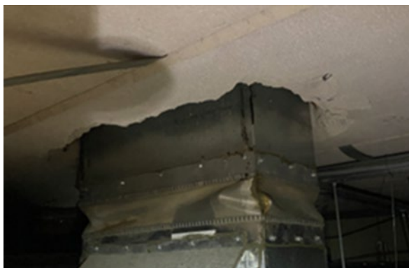
Figure 3.9 - Edge of RAAC plank site cut to fit outturn dimension
