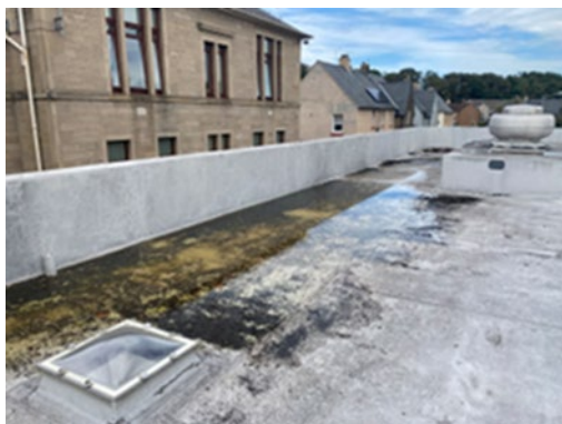
Figure 3.7 - Water ponding on roof
