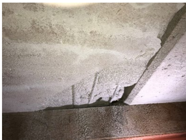
Figure 3.1 - Distressed end bearing
