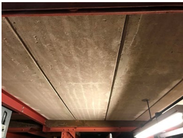
Figure 3.3 - Soffit discolouration indicating low cover
