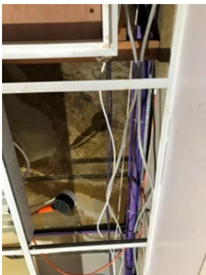
Figure 3.6 - Chronic water penetration to slab soffit
