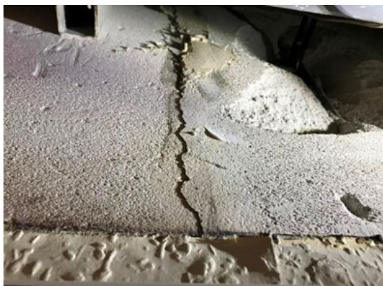
Figure 4.9 - Cracked infill joint between partitions
